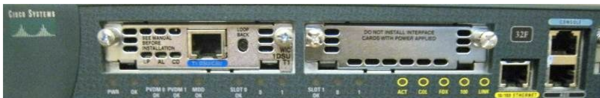
Figure 1.3 – Modular Cisco Router with a Blank Slot to the Right
