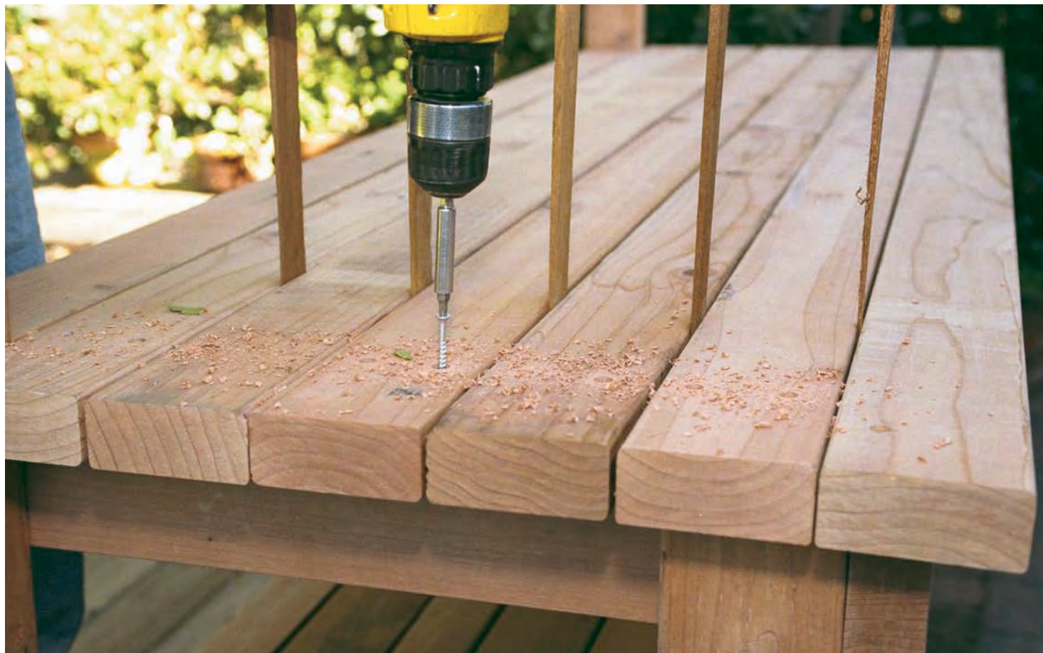
Evenly space the upper- and lower-shelf boards. Use shims as spacers and to keep the boards in place while driving in the deck screws.
