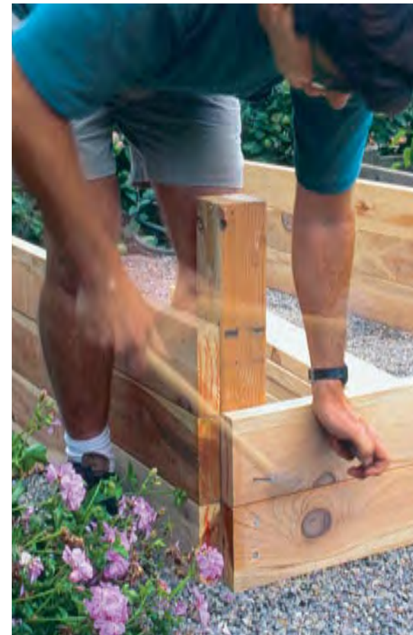
Pull it all together. Stand up the constructed long sides of the bed so that they are 4 ft. apart and parallel to each other. Complete the bed by nailing the short 4-ft.-long 2x6 boards to the posts.
