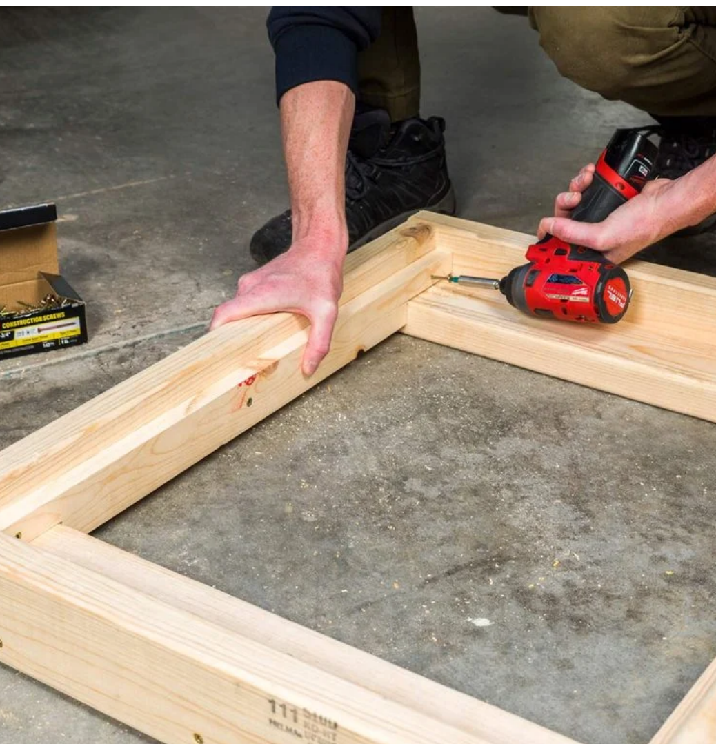
Rip the 1×3 to 2-in. wide on the table saw and crosscut to the length stated in the Cutting List. Cut a 1-in. deep x 3-1/3-in. wide notch at both ends with the jigsaw of the 2-in. wide boards to create the mounting strips (D). Glue and screw the mounting strips to the inside
